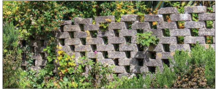
Inappropriate concrete wall
