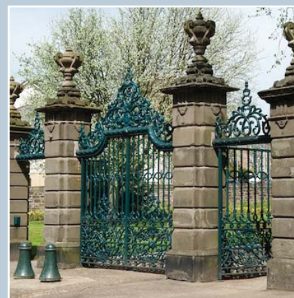
Baxter Park, Dundee. The cast-iron gatepiers and cresting of 1863 survived, but the gates were missing until they were replaced as part of the restoration of the park in 2007.
