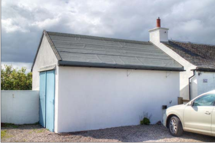
Inappropriate felt roof
